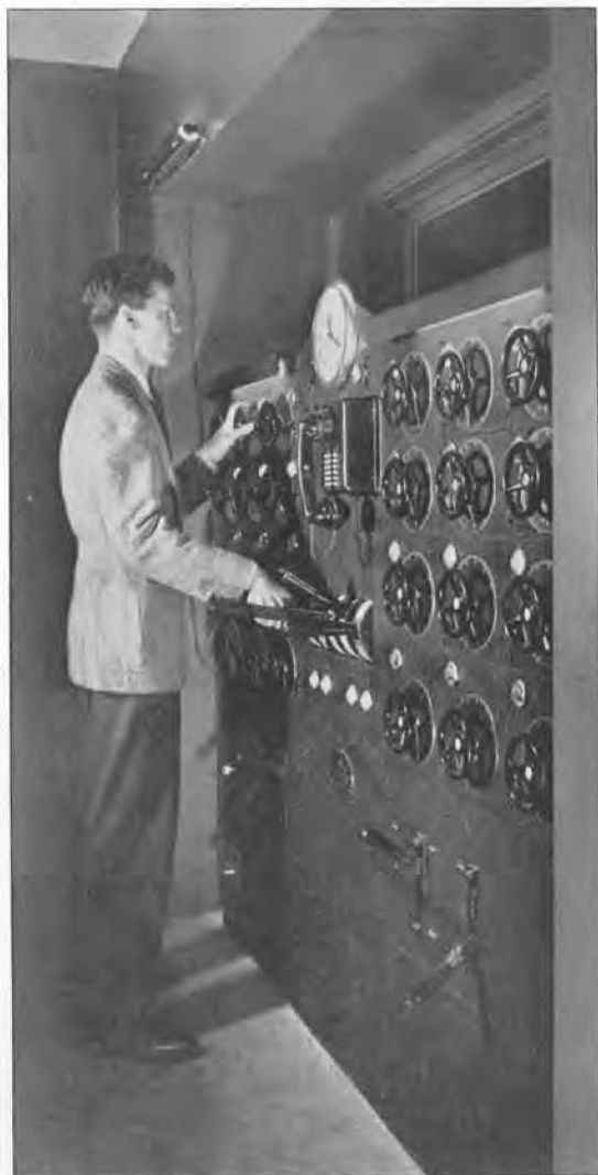
VARIACS in a theater lighting control panel at Allegheny College.
